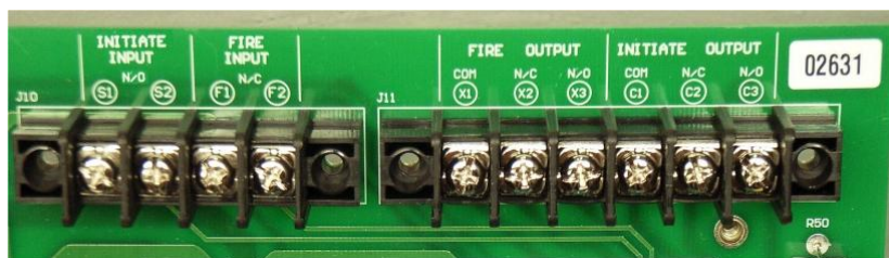
Input & Output control wiring terminals
