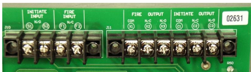
Input & Output control wiring terminals
