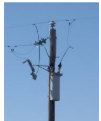
A 240V tap on a Single Wire Power line
